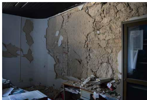
Figure 2: Office inside Colonia IX Maggio, abandoned after 2009 earthquake (Photocredit: E. G. De Leon)
